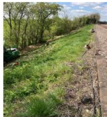
Where the de-veg team were working at the bottom of the embankment (approx. 11m from running line)
