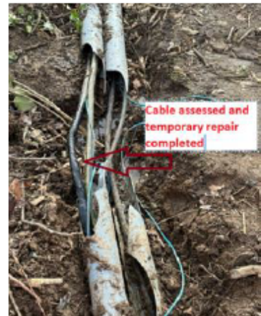
The damaged pipe
