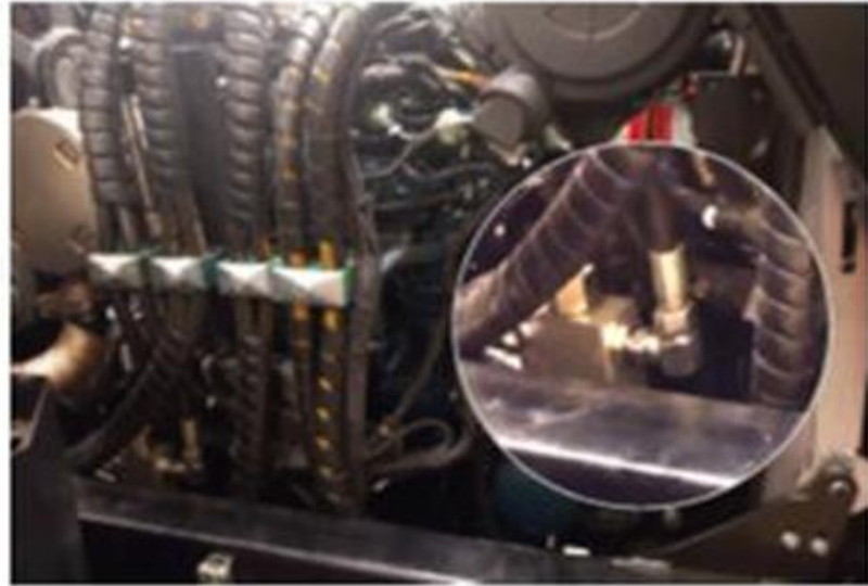
Old position of over centre valve
