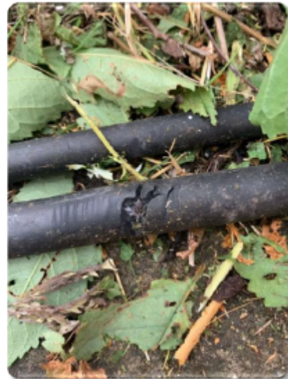
Damaged 10-core cable
