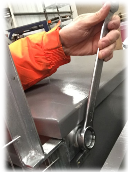
Figure 17 – Remaining M20 Bolts
