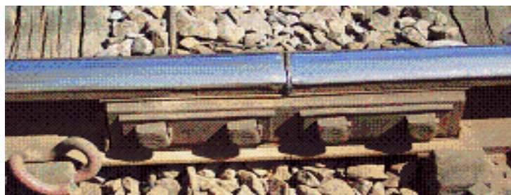
Figure 4 – Incorrect sleeper spacing
