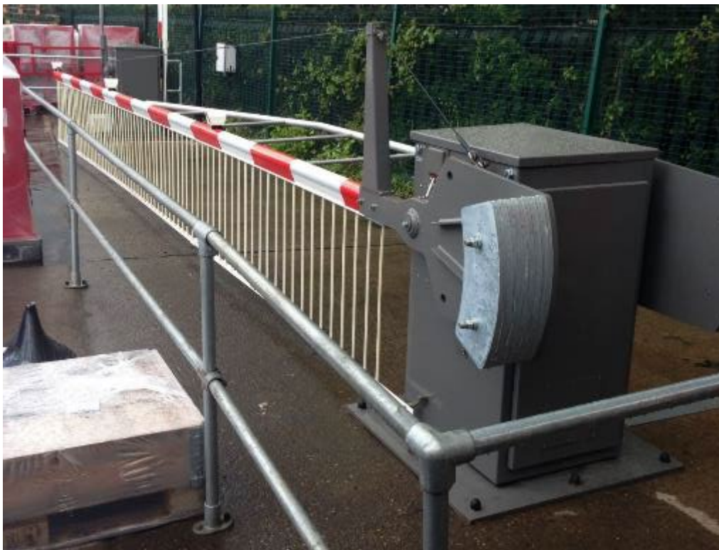
Figure 1 - Newgate Barrier Machine - NGR18000
