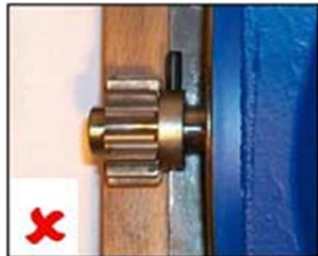
Figure 6 – Spirol pin working loose
