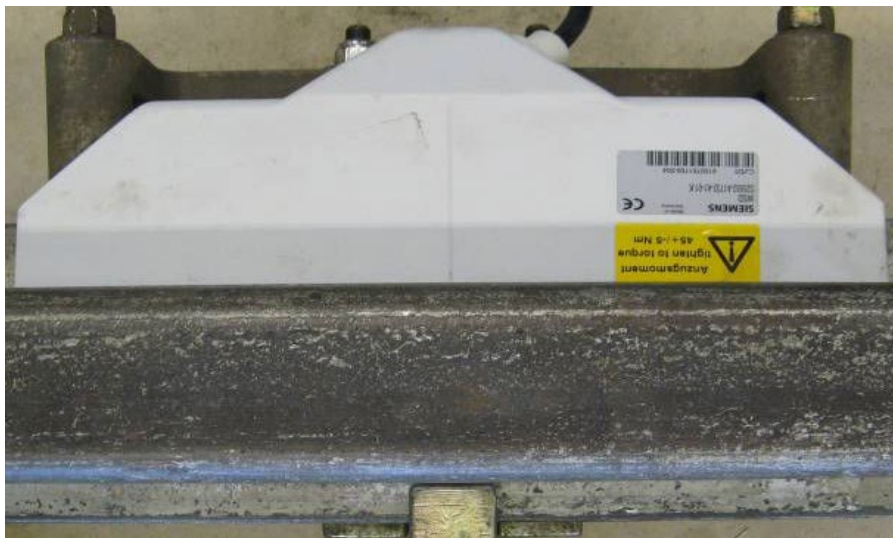
Figure 2 – Too close to the rail
