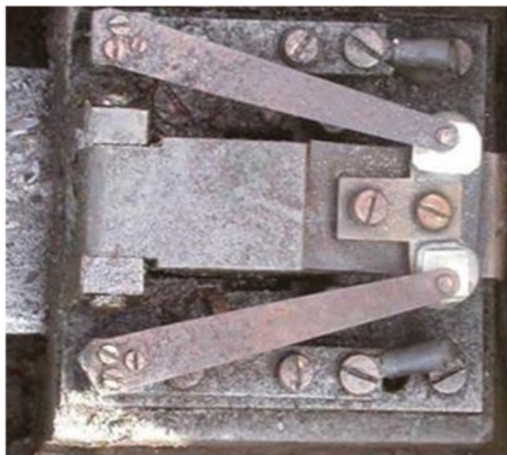
Figure 3 – Bridge Bold Detection
