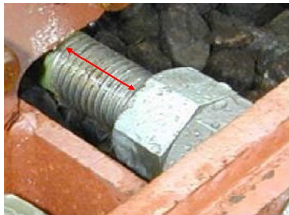
Figure 13 - Example of visible thread showing after installation of hardlock nuts. 11 threads showing.
