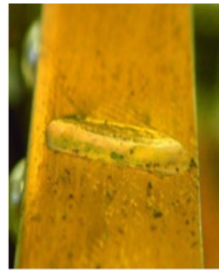
Figure 3 – Defective Level of Damage
