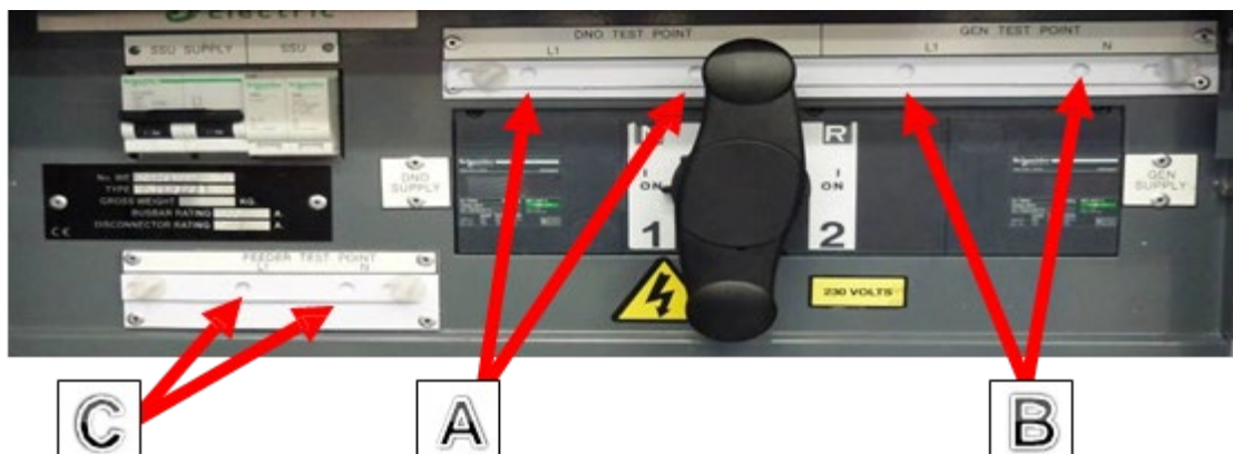
Figure 4 – Feeder Power Supply
