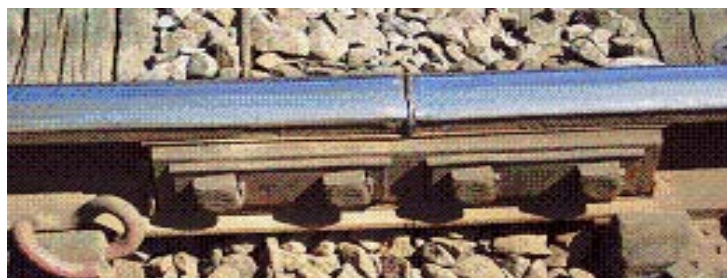
Figure 4 – Incorrect sleeper spacing
