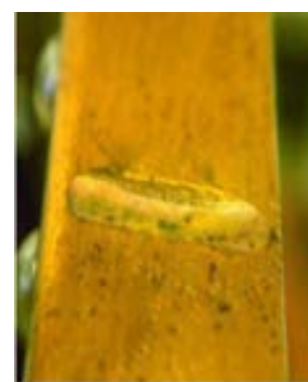
Figure 6 – Defective Level of Damage
