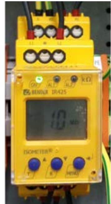
Fig. 11. Earth Leakage Detector
