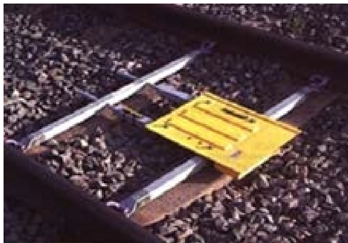
Figure 1 - TASS Balise assembly installed using the rapid fixing kit
