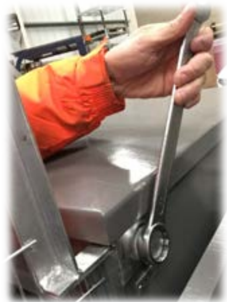
Figure 17 – Remaining M20 Bolts
