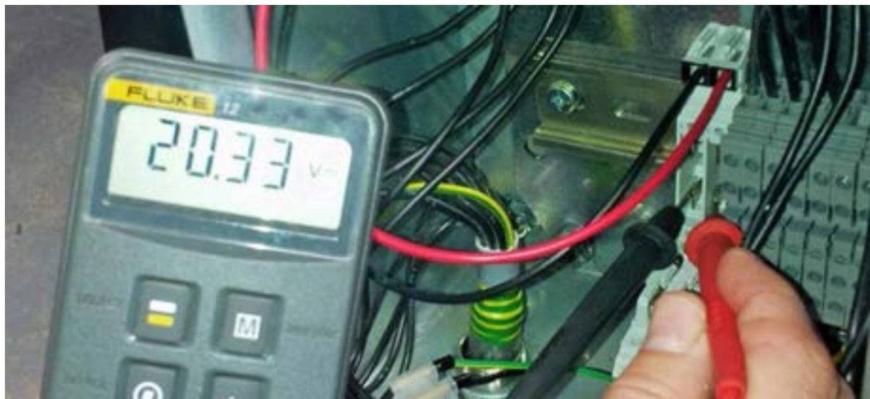
Figure 8 - Solar Panel incoming terminations
