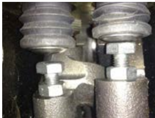
Figure 18 – Micro-switch bellows damage
