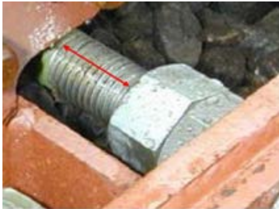
Figure 13 - Example of visible thread showing after installation of hardlock nuts. 11 threads showing.
