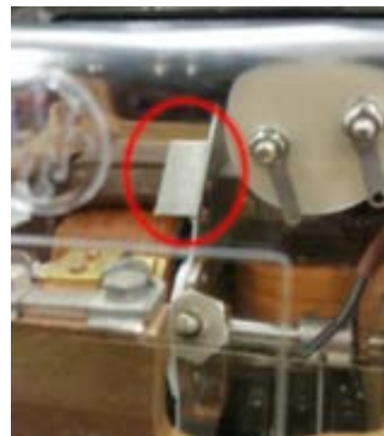
Figure 4 – Vane in the Energised position
