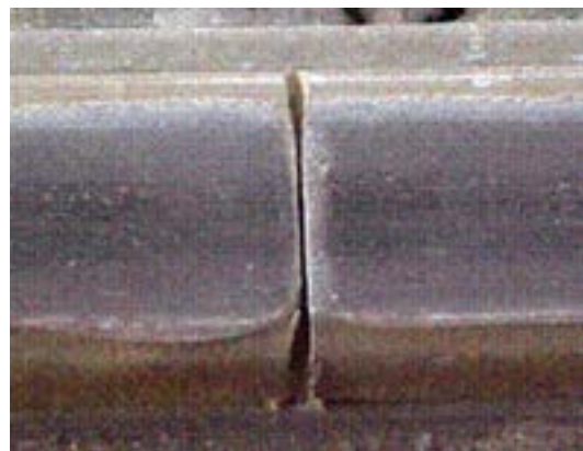
Figure 7 – End Post Missing
