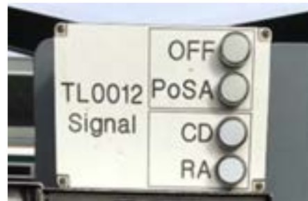
Figure 1 – Dispatch Interface Units
