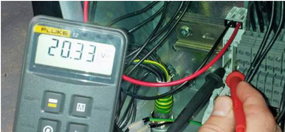
Figure 5 – Solar Panel Voltage Measurement
