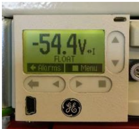
Figure 1 - Rectifier Controller Module
