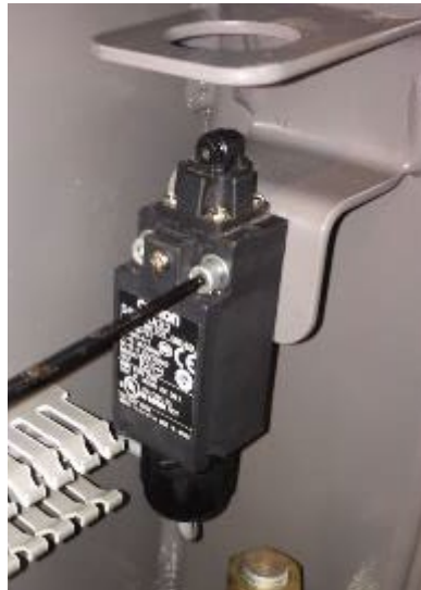
Figure 1 - Locking Pin Safety Switch
