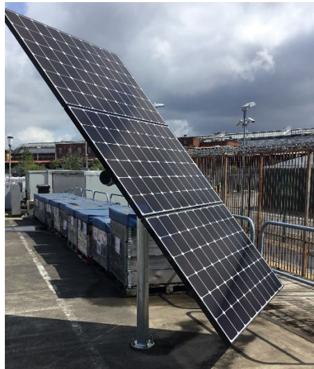
Figure 1 – A Three Panel Solar Array
