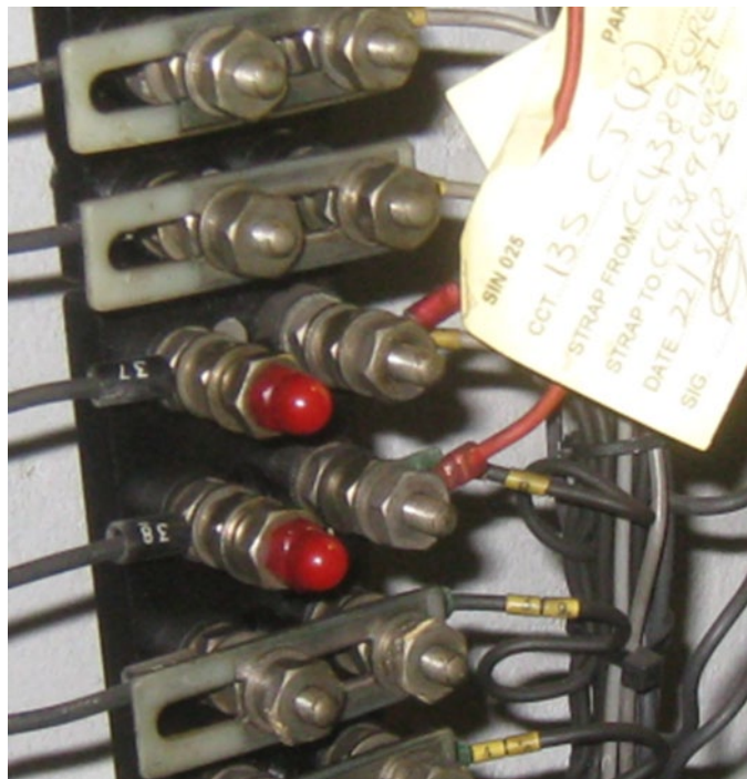
Figure 2 - Diversion Applied to a Terminal Block
