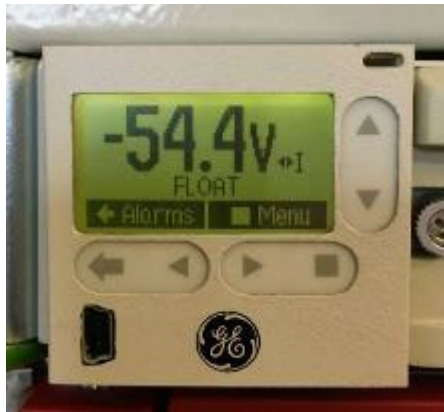
Figure 1 - Rectifier Controller Module
