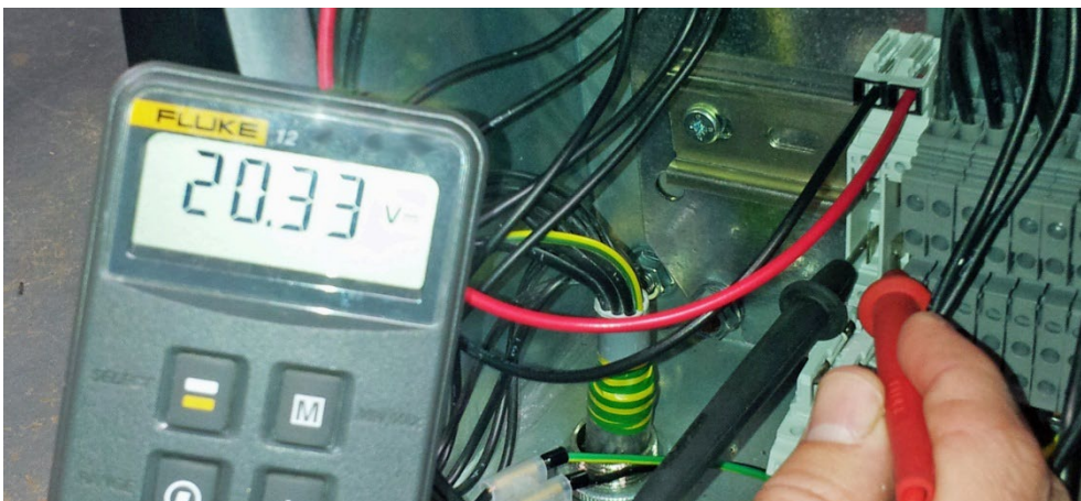
Figure 10 - Solar Panel Voltage measurement
