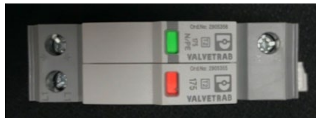
Figure 2 - Visual indication of an operational (green), and a blown Surge protector (red).
