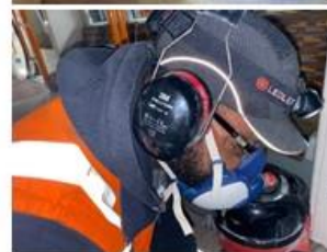
Wrong PPE for task
