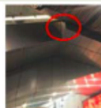
The location of panel prior to it falling .
