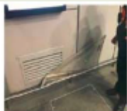
The triangle panel that fell into the public concourse
