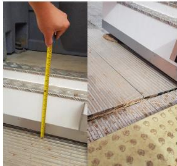
Images show steps at above 250mm (390mm) and uneven walkway
