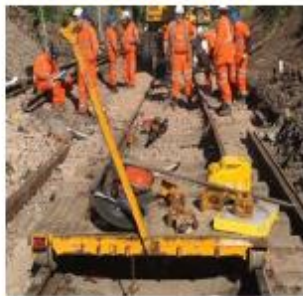
No push handles in place:
