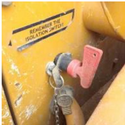
Isolator Key to be removed.
