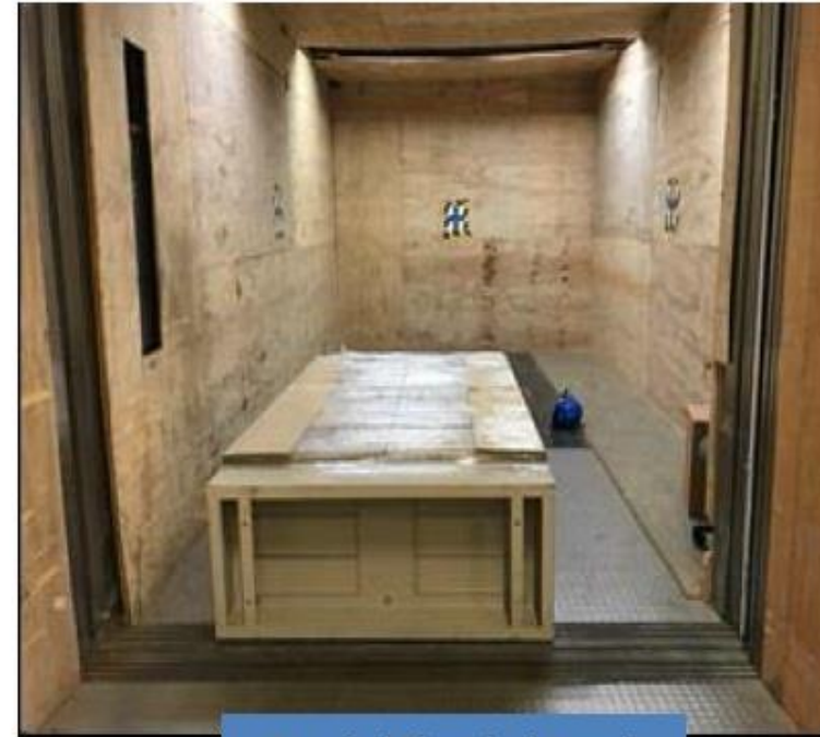
Topped Electrical Panels
