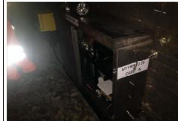
Location case with door missing
