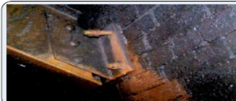
Photograph of failed stud
