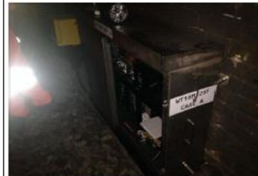
Location case with door missing
