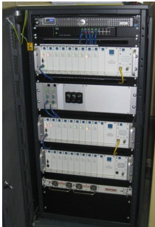
Figure 1 – RETB System Control Radio Rack
