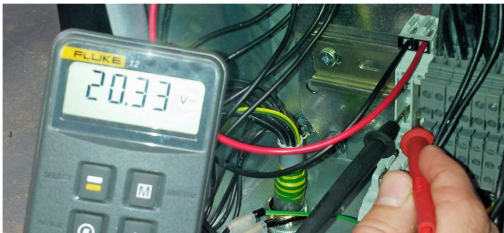
Figure 10 - Solar Panel Voltage measurement
